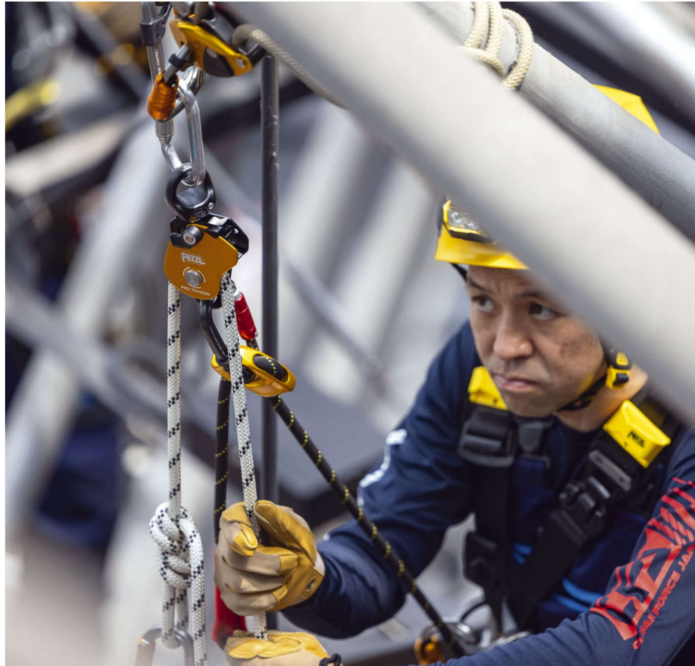
Rope access work at the Tokyo Metropolitan Theater © 2025 Petzl Distribution - Lafouche Tokyo Metropolitan Theater - Clean Force Japan
